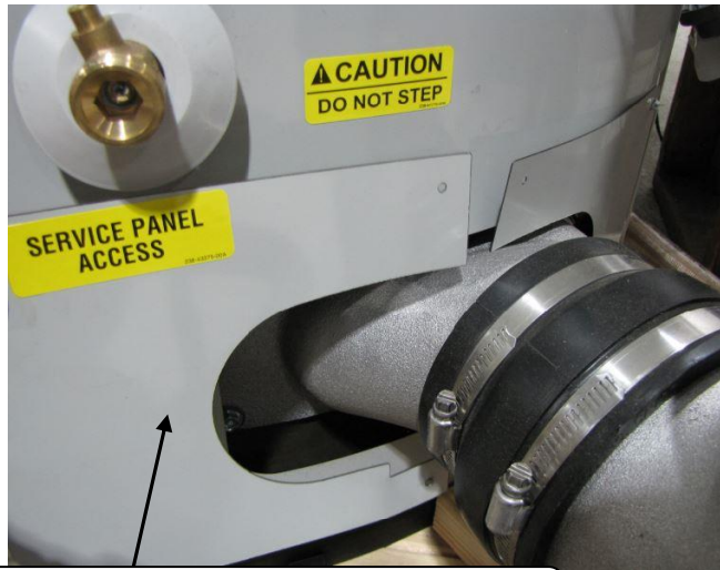
Exhaust tube pressure tap located behind service panel access doors at bottom of heater
